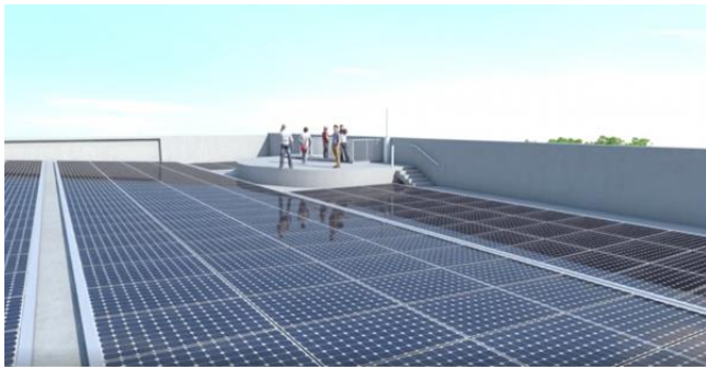
Solar Panels on Rooftop of NUS SDE4. Photo credit: SJ Sustainability.
